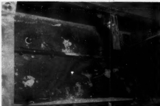
PAN FEEDER loading under the primary crusher is controlled by a small photoelectric cell.
